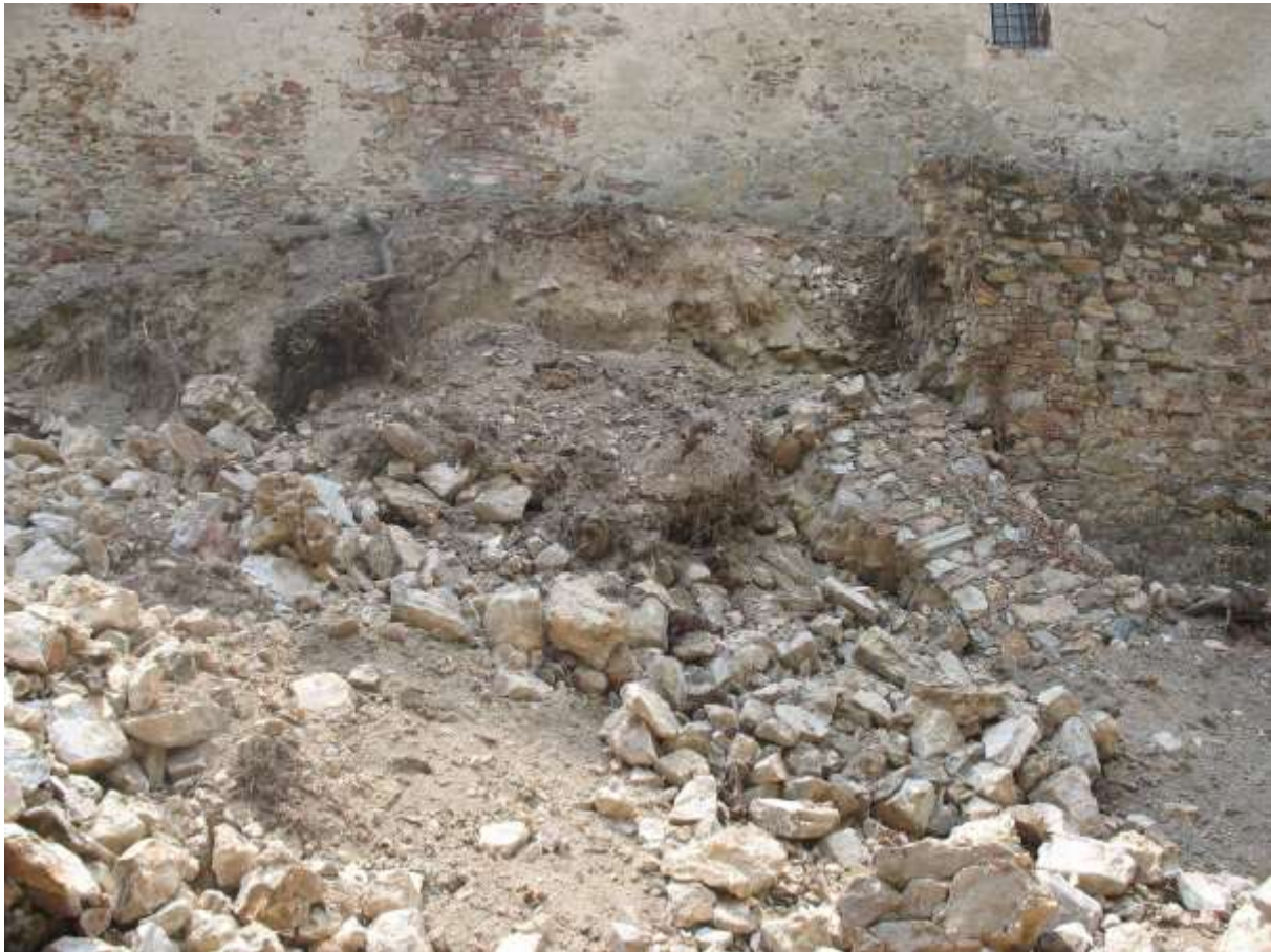
Fig. 2: Eskarp collapse of a retaining wall on the north side of the ditch (From: Ing. Michal Vondrák, 2012)
